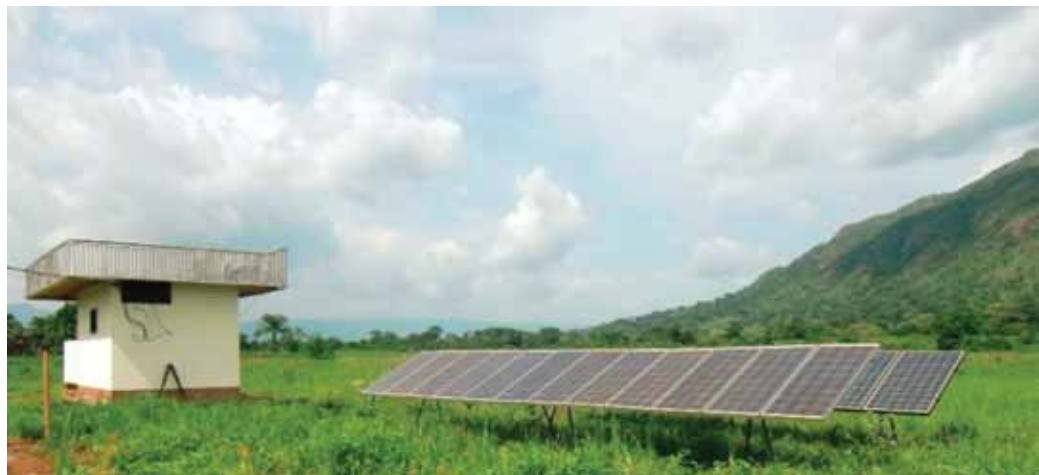
REI's pioneering Sabongari Power Station (May 2013)
